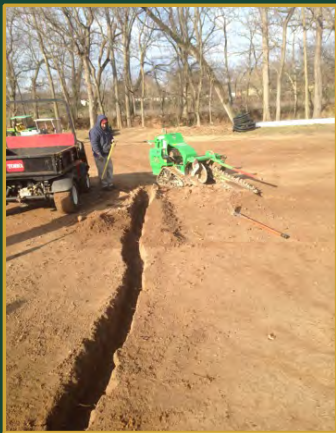
Chipping Green Drainage
